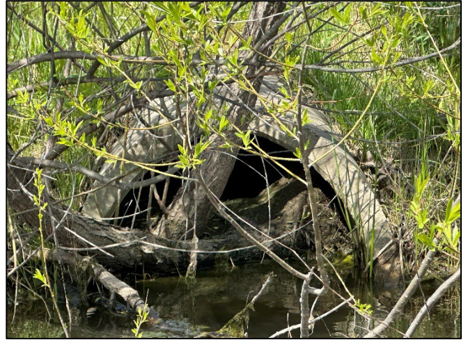
Photo 10. Tree growing in Pond 1 West Culvert
