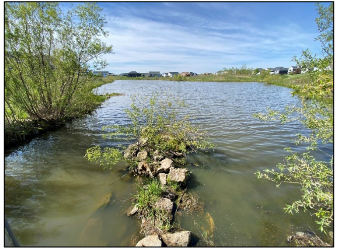
Photo 4. Rocky projection at inflow culvert, Pond 1
